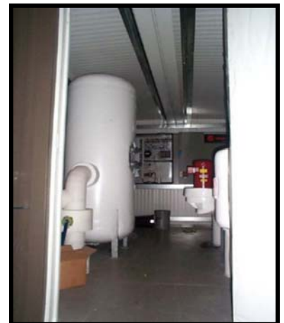
Pump house interior with chiller control panel
