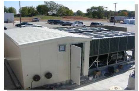
Custom Industrial Air-Cooled Chiller Package AFTER
