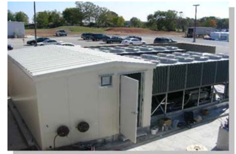
Custom Air-Cooled Chiller Package AFTER
